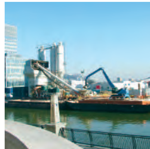
Location: Canary Wharf Hanson UK supply – All material (aggregates by barge) Capacity: 120m 3 per hour
