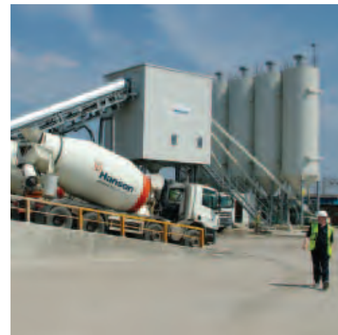
Location: Stratford City Hanson UK supply – All material Capacity: 140m 3 per hour
